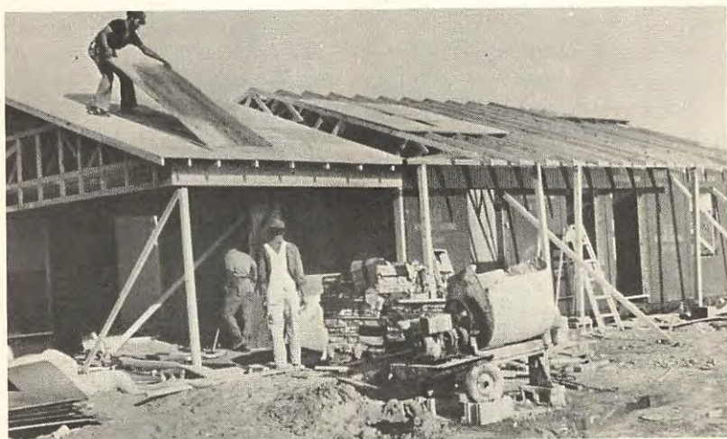
Workmen build one of the first two houses in the Lonoke subdivision.
