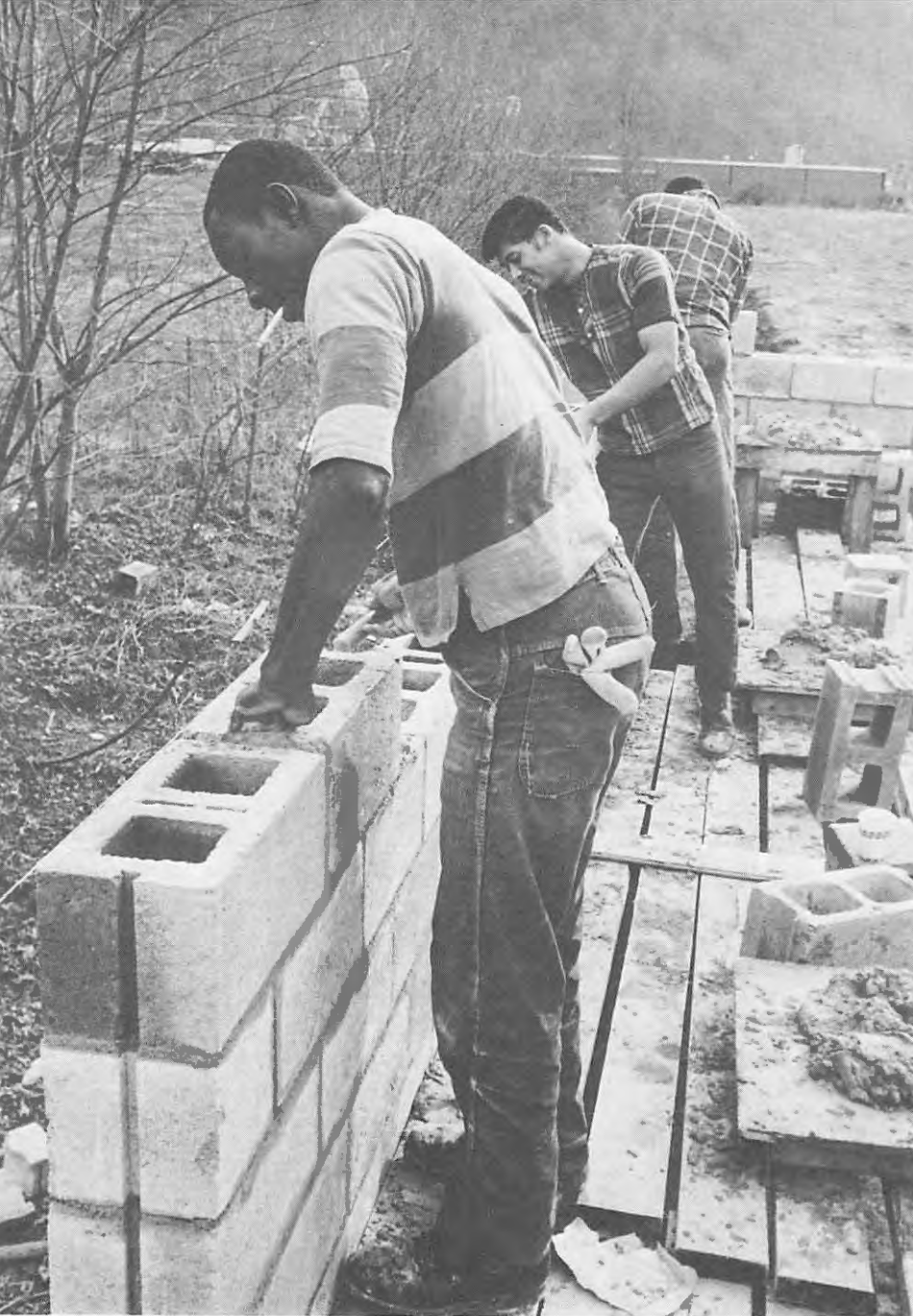
Job Corps trainees work on a community center for Indians on a reservation near Cherokee, North Carolina.
