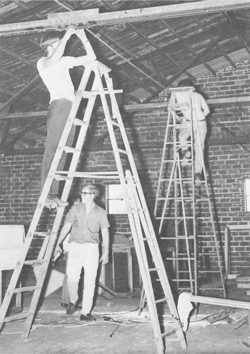
Students install electric wiring as local volunteers wind up their work of converting an abandoned warehouse into a museum in Caruthersville, Missouri.
