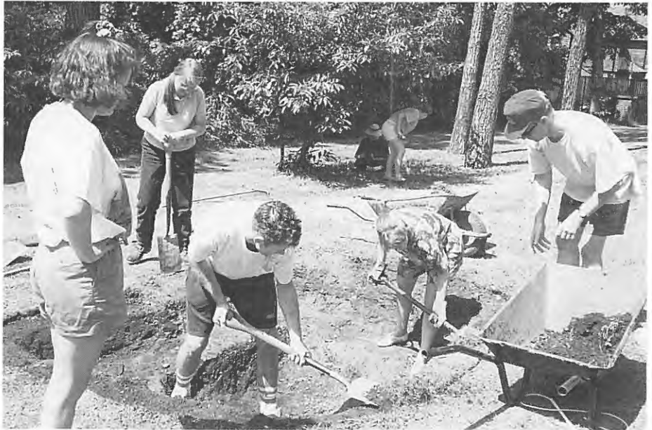
Sun Microsystems volunteers at a "pond digging" to create a fountain for Pinehurst Resource Centre (for the elderly) in Camberley, Great Britain.
